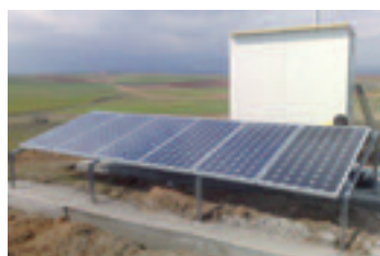
Solar Photovoltaik Telekommunikationssystem Solar photovoltaic telecom system
